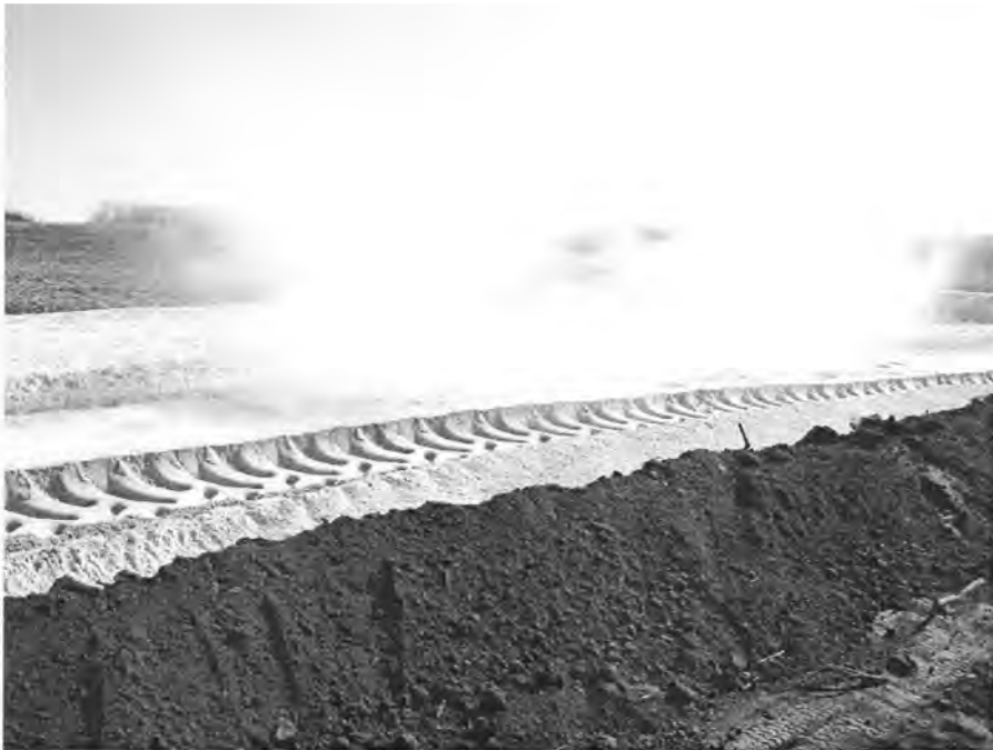
Figure 181. Steam Arising in Test Section One After Mixing Due to High Heat of Hydration
