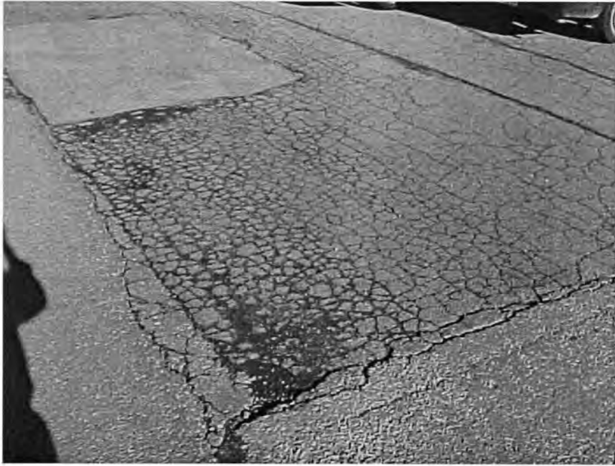
Figure 15. Alligator Cracking with Large Patches
