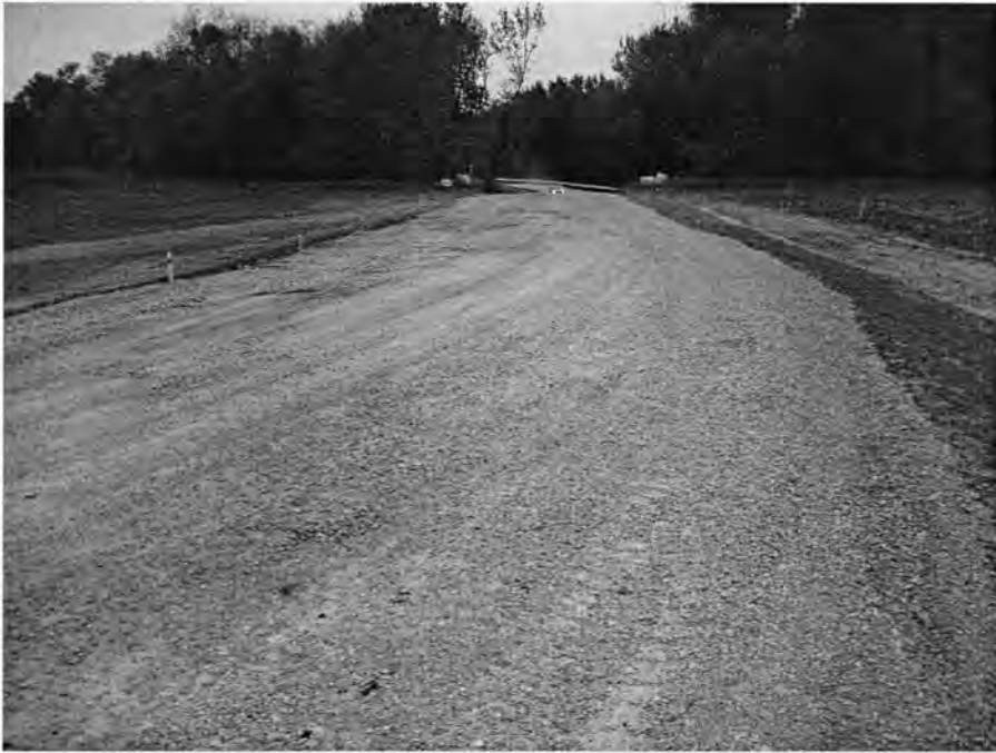
Figure 197. Control Section One (Foreground) and Control Section Two (Background) on April 30, 2004
