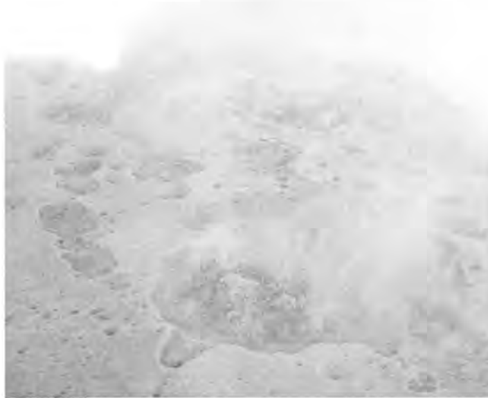
Figure 182. Water Vapor Causing Bubbling of Material before Compaction
