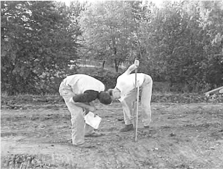
Figure 216. DCP Testing on Westbound Entrance Ramp of I-235 at 35th Street in West Des Moines
