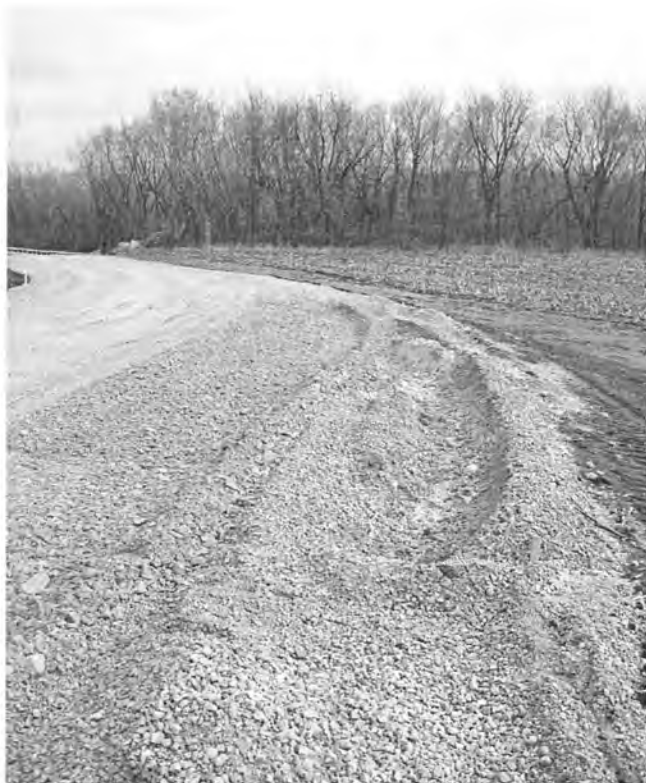
Figure 190. Extensive Rutting in Test Section One on March 2, 2004
