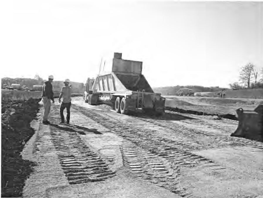
Figure 67. Placement of Fly Ash in Test Section Two with a Bottom Dump
